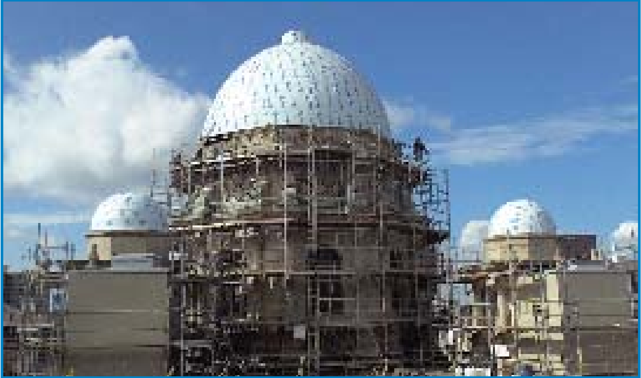
A view of the work being done on the Onondaga County Courthouse domes in Syracuse, New York. SOPREMA's Lastobond Shield HT is being used on the main dome and two smaller domes to protect the structure from ice, snow and rain damage. The courthouse was built in 1907.
